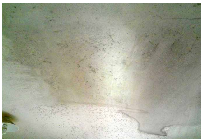
Above: Mould in one of the whānau’s homes.
