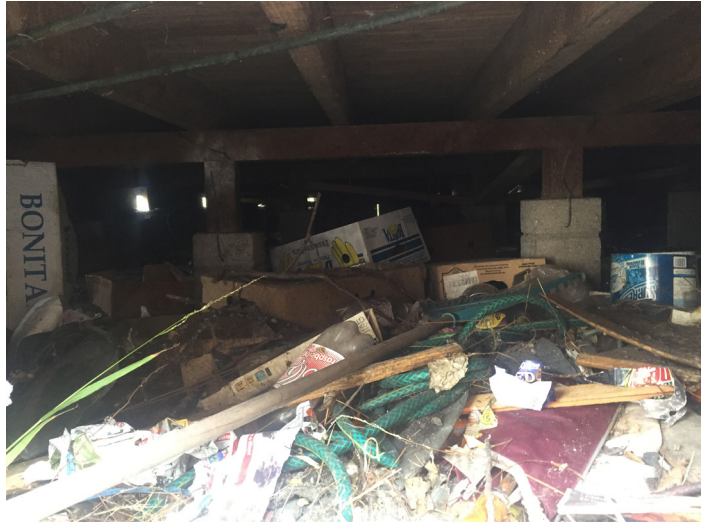
Left: The lounge wall had rotted from the roof leak. Above: No groundsheet or underfloor insulation. There is space to install both, but under the house needed clearing.
